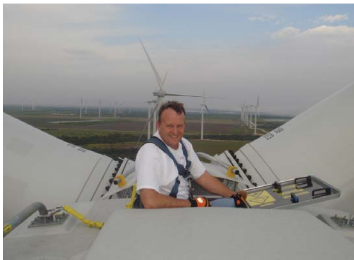
System 3 Inc. founder Tom Wilbert working on a wind turbine tower at the Roscoe Wind Farm in Roscoe, Texas.
